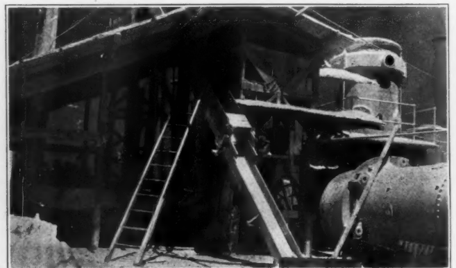
Lime Hydrators at Top of Sand and Gravel Plant
